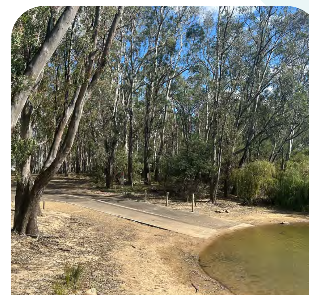
Boat Ramp Infrastructure - safety & access issues
